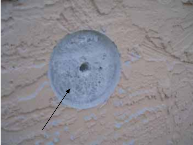
Core samples were taken at locations previously described as uneven & not appearing to be the correct depth.
