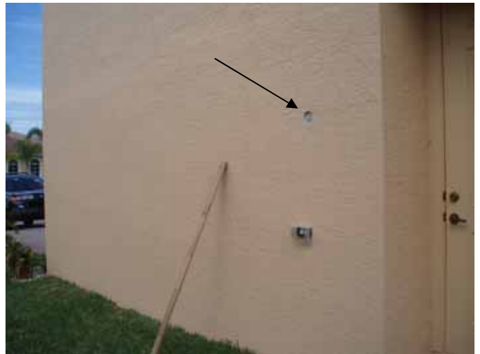
Location of the next photo at the west side of the house. Core samples were taken & the thickness of the stucco was measured at each sample.
