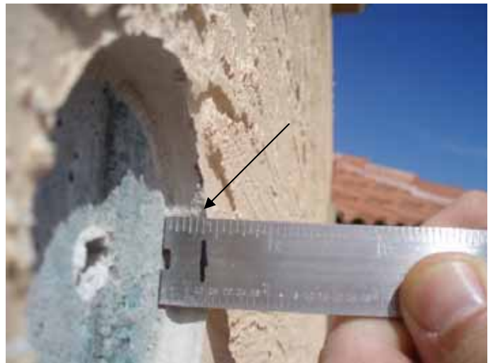
Core samples were taken & the thickness of the stucco was measured at each sample. The thickness of the stucco was 3/8 " at this location.
