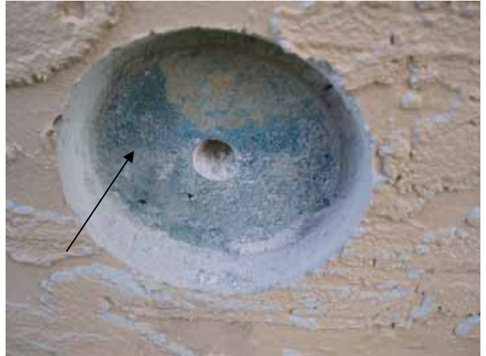
The blue coloring is the bonding agent applied to the exterior wall prior to the stucco installation.
