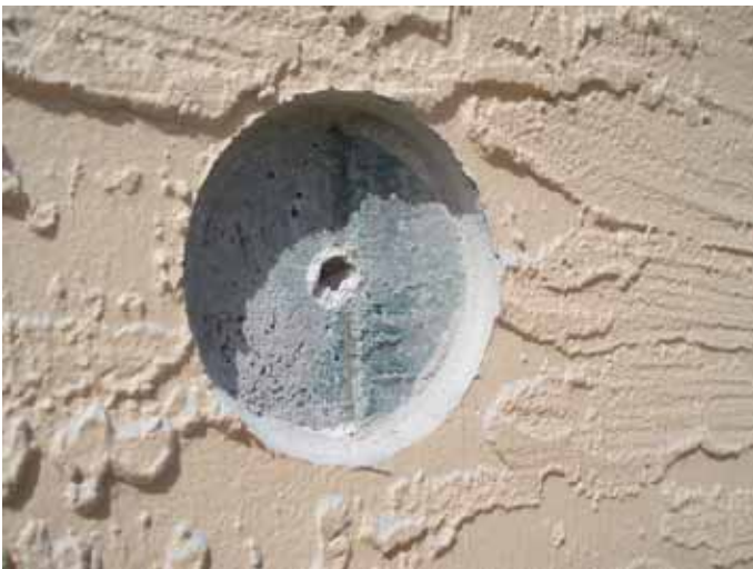
We were asked to take core samples to help determine the thickness of the stucco at areas previously identified in the home inspection report dated 03.10.07
