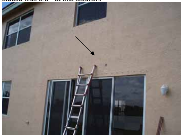
Location of the previous photos at the back of the house over the sliding glass doors.
