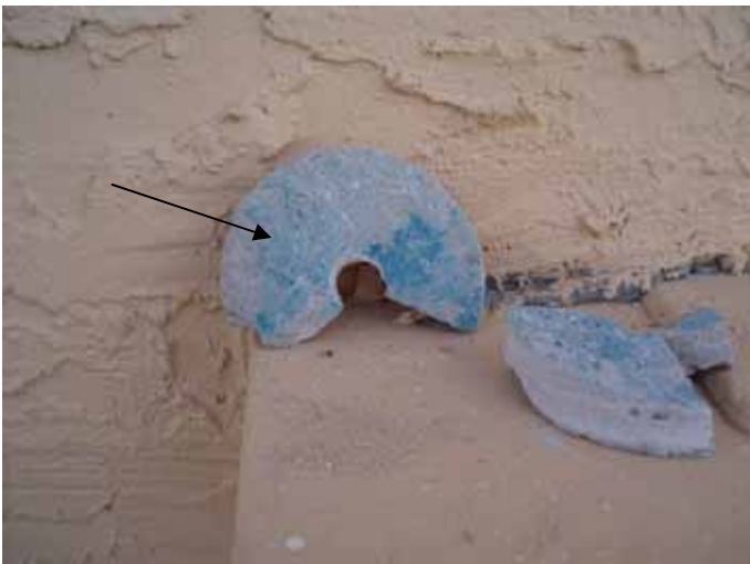
The blue coloring is the bonding agent applied to the exterior wall prior to the stucco installation.
