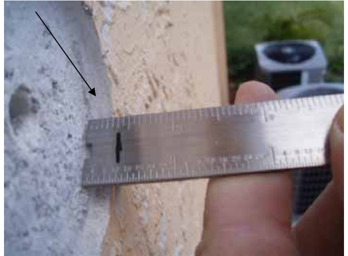
The stucco measured 5/16" at this area. The stucco should be applied to a thickness of 5/8".
