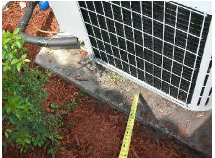
The A/C condensers are not secured properly. There are not enough straps at the base of the unit. M301.13.1
