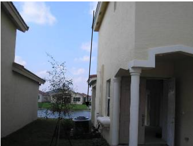
Gutters have been installed in accordance with the manufacturer's installation instructions. §M304.1
