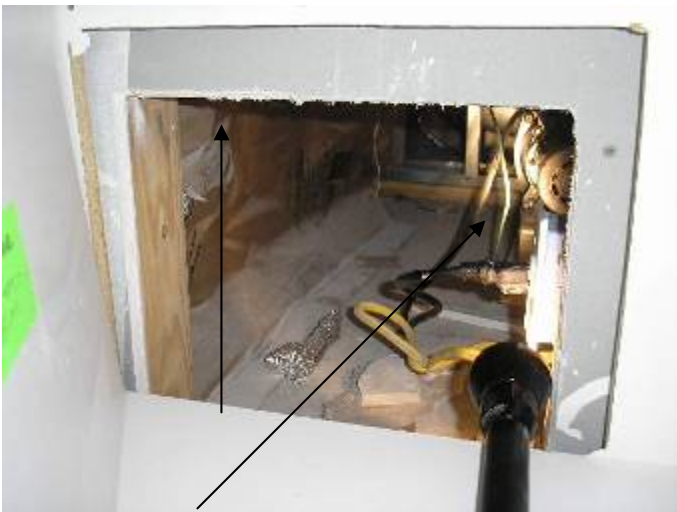
The opening in the cabinet is not big enough to allow the whirlpool tub pump motor to be accessed for service.
