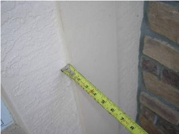
We recommend core sampling to verify the thickness of the exterior stucco & compliance with ASTM C 926.
