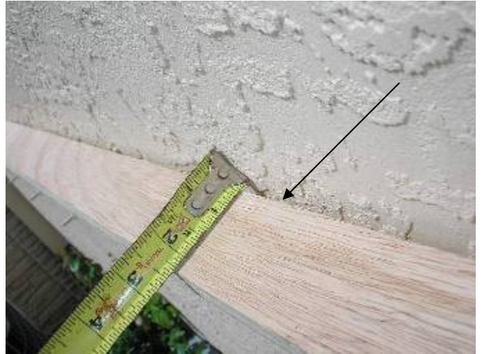
The stucco at some at the walls is concave or curved in & does not appear to be the correct thickness. §2509.1.1, ASTM C 926
