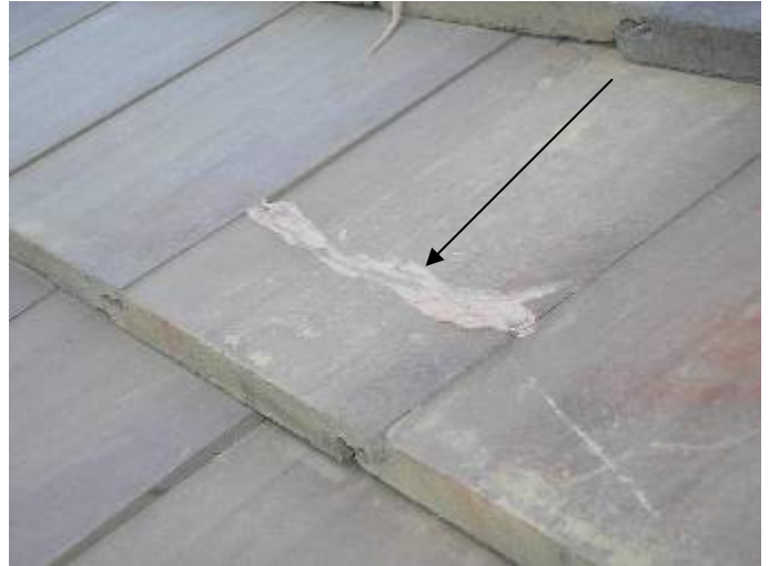
There were broken & incorrectly repaired roof tiles at several locations. The broken roof tiles should be removed & replaced, not "glued" back together.
