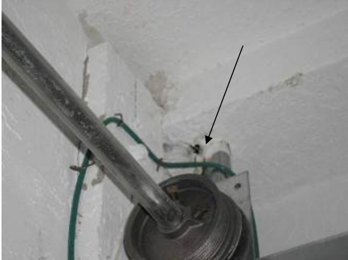
There are unsealed holes & openings in the drywall around the piping penetrations through the ceiling. The openings need to be sealed as required.
