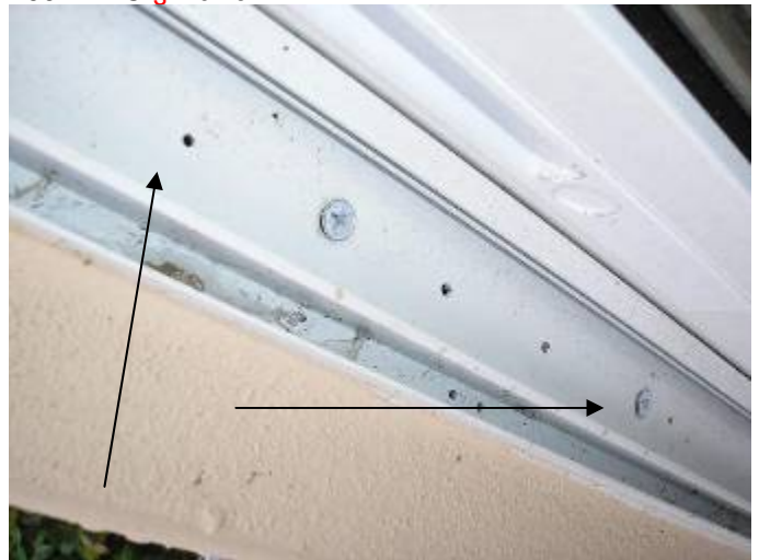
Some of the screw anchors & openings are not completely set & not sealed to prevent water & pest intrusion at sliding glass door frames. 13-606.1.ABC.1.2
