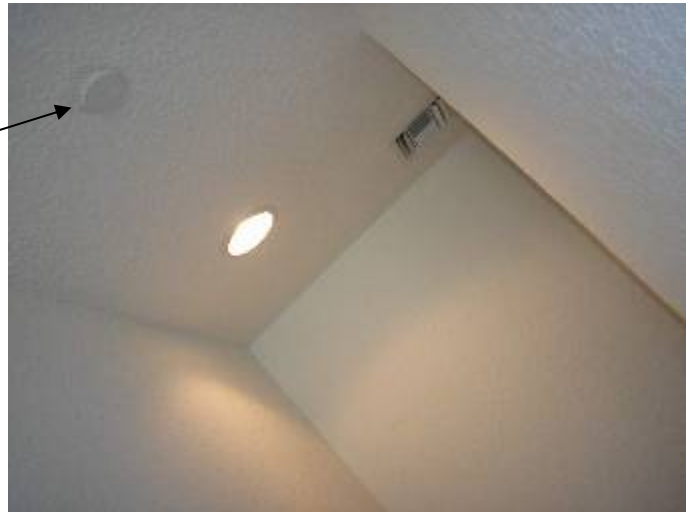
The fire sprinkler cap appears to be sealed in place & would not work in the event of an emergency at the 2 nd floor stairwell ceiling.
