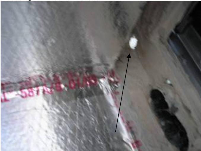
The ductwork is not completely sealed at the return air plenum under the AC air handler. §M603.1
