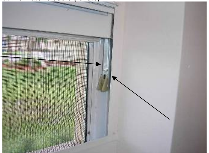
The balance rod is not working correctly at the first floor bathroom window.
