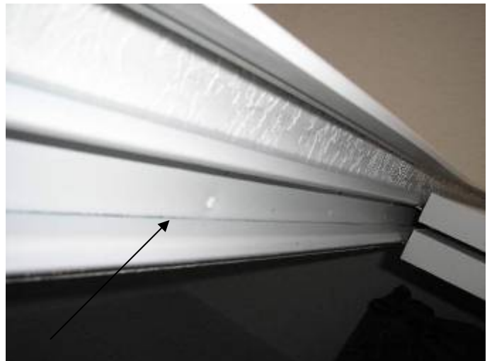
Some of the anchor screws are not installed at the upper track at the mirrored bypass closet doors.
