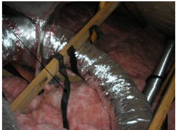
Some of the ductwork was not correctly supported off the attic insulation or other ductwork to prevent condensation & related problems. §M603.11, §M603.5.6.6
