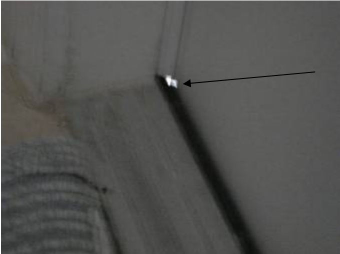
The door & frame are not completely sealed at the front entryway. §13-606.1.ABC.1.2
