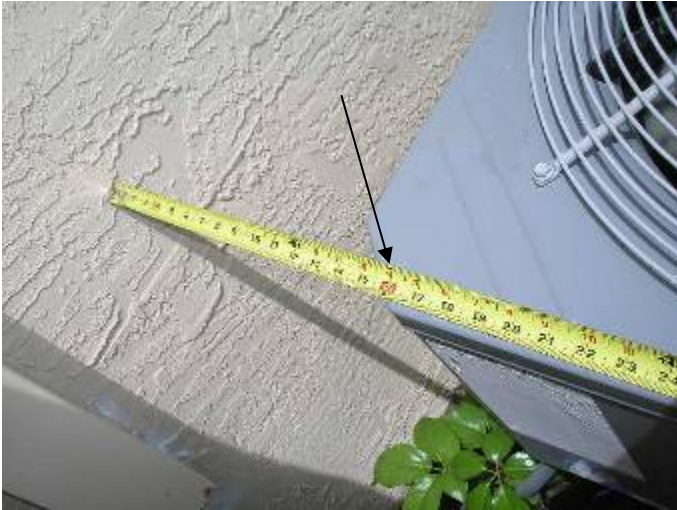
The AC condensing unit is turned the wrong way. 36 " working space clearance is required at the electrical access panel covers. 2002 NEC §110.26
