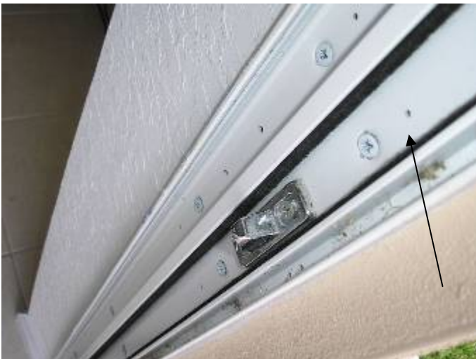
Some of the screw anchors & openings are not completely set & not sealed to prevent water & pest intrusion at sliding glass door frames. 13-606.1.ABC.1.2
