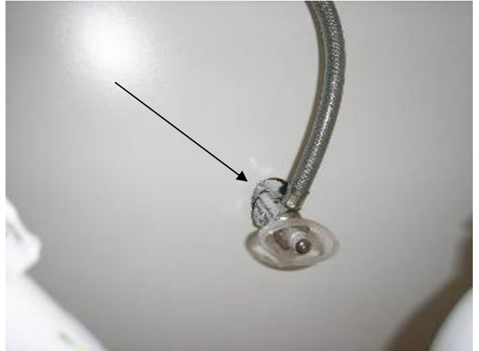
Some of the plumbing pipes have loose, unsealed or missing escutcheons (covers) inside the sink cabinets.
