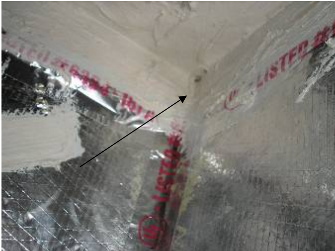
The ductwork is not completely sealed at the return air plenum under the AC air handler.
