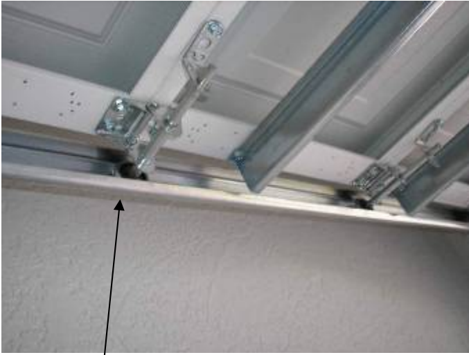
The rollers at the garage vehicle door are very noisy & not operating correctly when the door is opened or closed.
