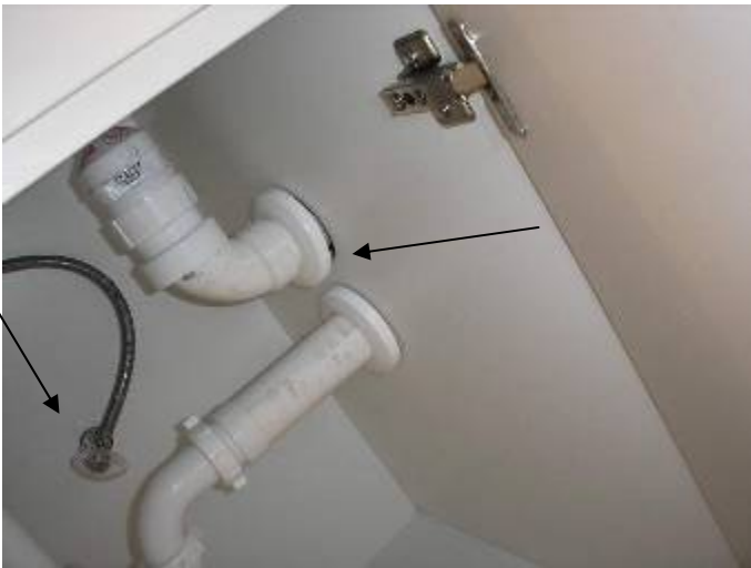
Some of the plumbing pipes have loose, unsealed or missing escutcheons (covers) inside the sink cabinets.
