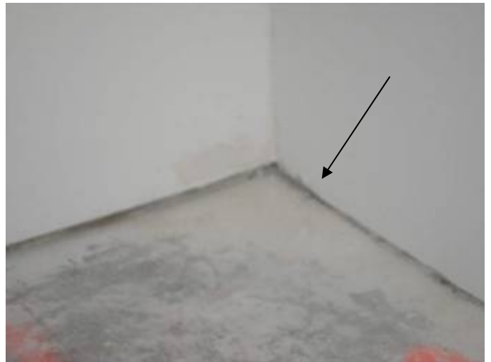
The walls are not sealed at the floor under the kitchen counters.
