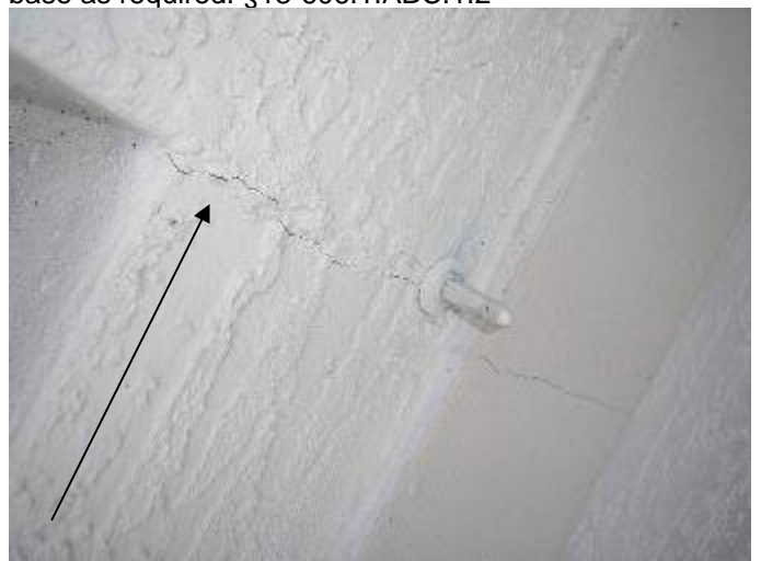
There are unsealed cracks in the stucco banding. §1403.1.3
