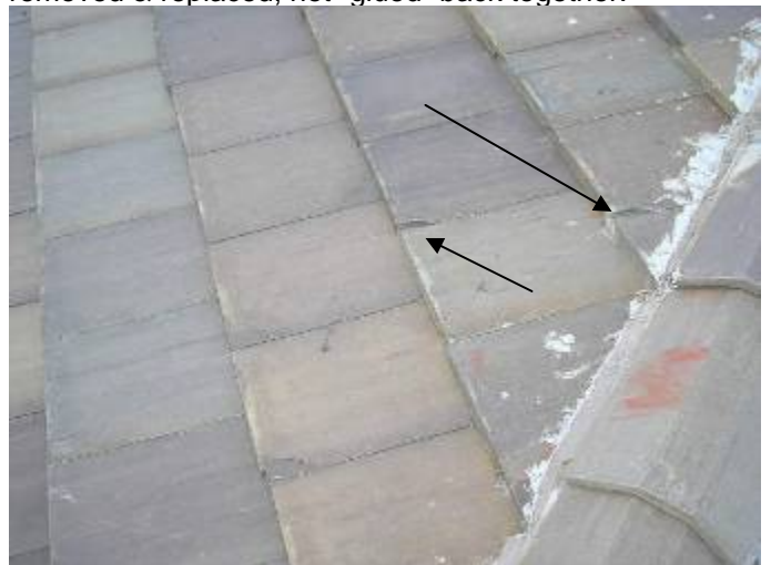
All loose & damaged tiles need to be correctly secured &/or replaced.
