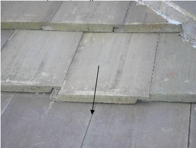
Some of the tiles are loose &/or have slipped out of place. All loose tiles need to be correctly secured.
