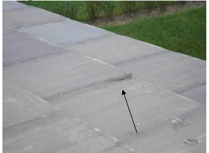
There were broken & incorrectly repaired roof tiles at several locations. The broken roof tiles should be removed & replaced, not "glued" back together.
