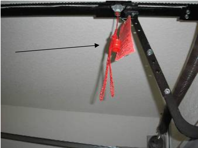
The red emergency release cord is located too high off the floor. The cord height should be 6' above the floor. See the manufacturer's installation instructions.
