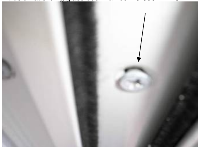
Some of the screw anchors & openings are not completely set & not sealed to prevent water & pest intrusion at sliding glass door frames. 13-606.1.ABC.1.2
