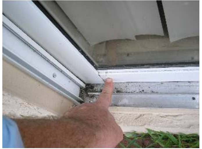
The south side sliding glass door did not open & close correctly.
