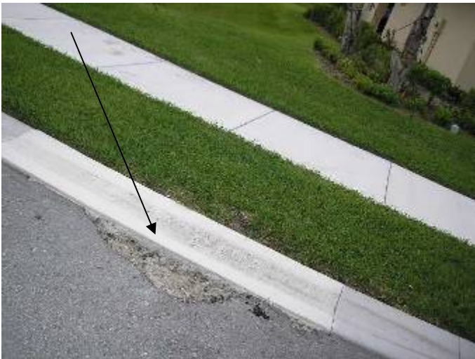
The damaged black top paving is a trip hazard at the street in the front of the house.
