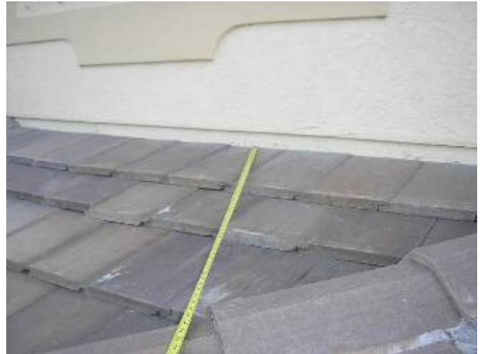
The roof wall abutments have not been correctly pointed up with mortar at the back patio. R118-3.13
