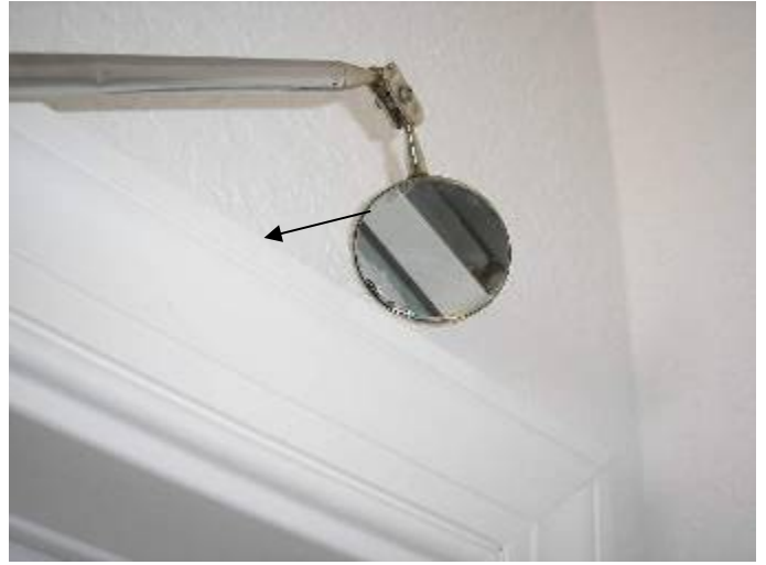
The side & tops of the garage/hall entry way door frame are not correctly sealed. §13-606.1.ABC.1.2
