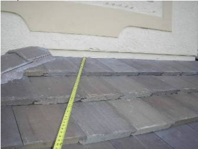
The roof wall abutments have not been correctly pointed up with mortar at the back patio. R118-3.13
