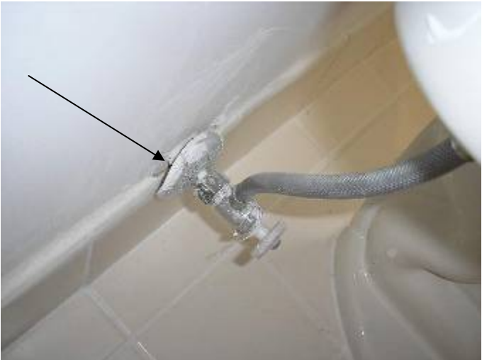
The plumbing supply piping is not correctly covered by the escutcheon at the master bathroom (W.C.) toilet.
