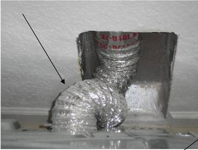
The thin aluminum foil dryer vent duct material is a fire hazard per CSPC & the manufacturer. See warning label on back of the dryer. §M304.1
