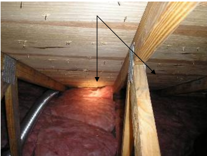
Some of the insulation is blocking the attic vent air circulation at the eaves. Baffle boards should be installed at all locations.
