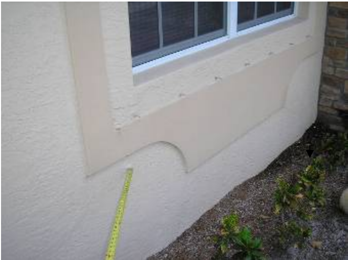
The stucco at some at the walls is concave or curved in & does not appear to be the correct thickness. §2509.1.1, ASTM C 926
