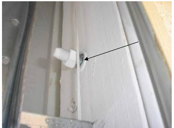
Some of the garage door buck anchor nuts are loose & not correctly secured. §1606.1.3, §2306.2
