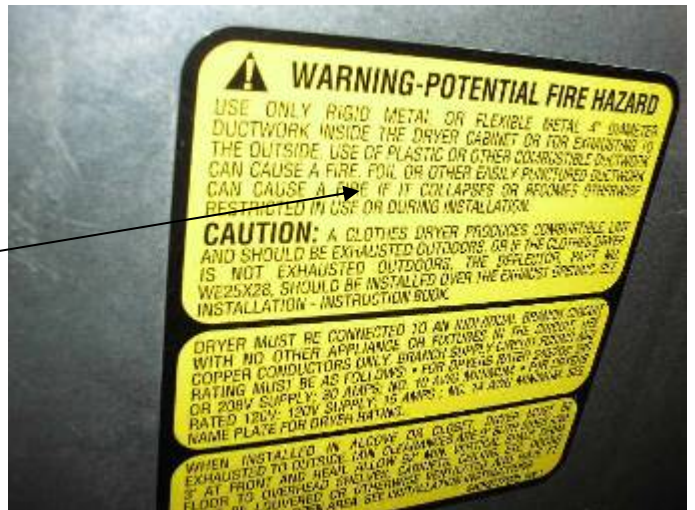
The thin aluminum foil dryer vent duct material is a fire hazard per CSPC & the manufacturer. See warning label on back of the dryer. §M304.1
