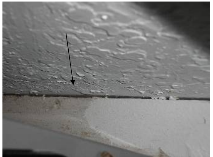
The AC mechanical closet is not completely sealed as required. §13-410.1.ABCD.3.7
