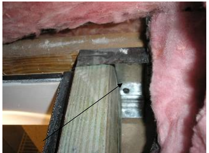
The light gauge framing metal & drywall screws are not designed or intended to be used for load bearing support at the 2x4 blocking at the attic access opening.
