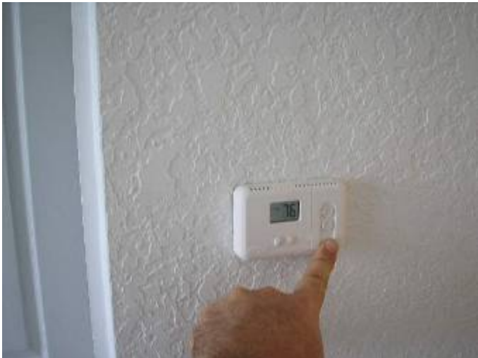
The thermostat did not operate correctly after the heat was turned on.
