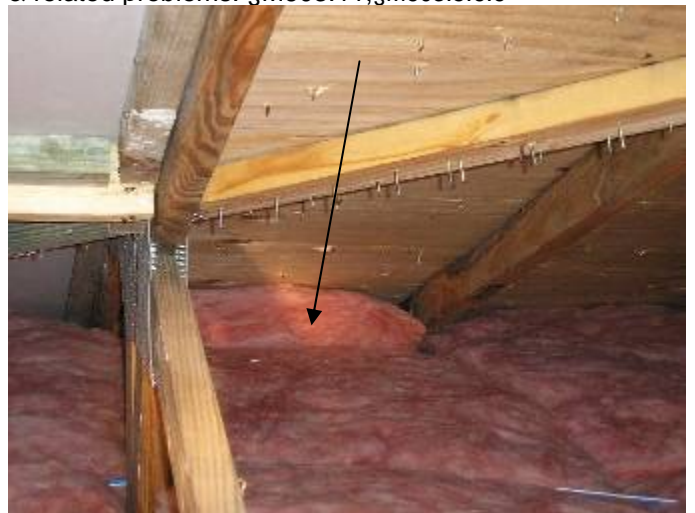
Some of the insulation is blocking the attic vent air circulation at the eaves. Baffle boards should be installed at all eave locations.
