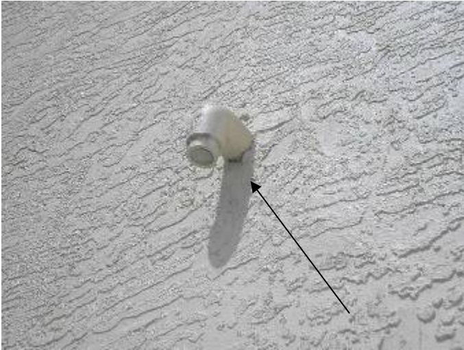
The stucco around the drain line is not completely sealed at the back of the house. §13-606.1.ABC.1.2, §1403.1.3.
