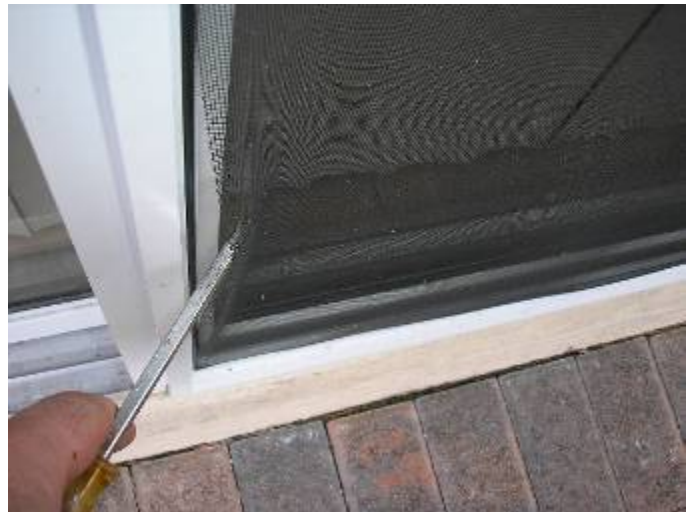
The screening is coming out of the frame at the rear sliding door.
