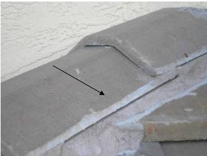
Some of the hip & ridge cap tiles do not appear to be correctly secured or bonded. §1518.8.5, §1518.8.11, 1507.4.5.2.1
