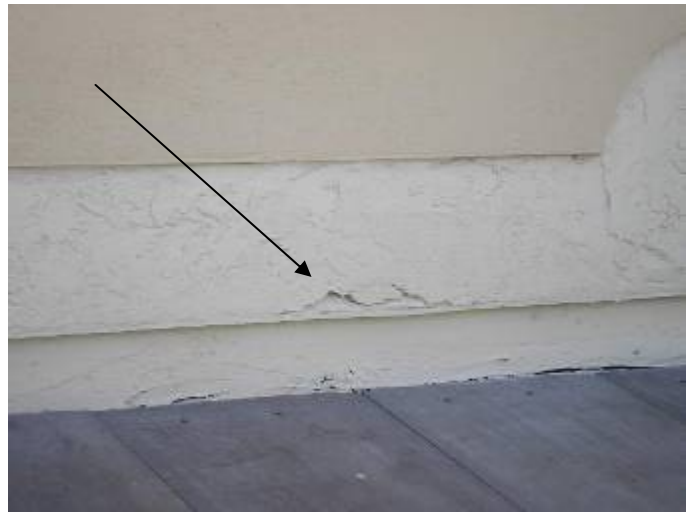
There is missing stucco above the garage roof tile at the 2 nd floor exterior wall. §13-606.1.ABC.1.2, §1403.1.3.
