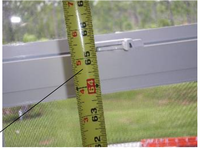
The window locks should not be higher than 54" above the floor in the bedrooms.
