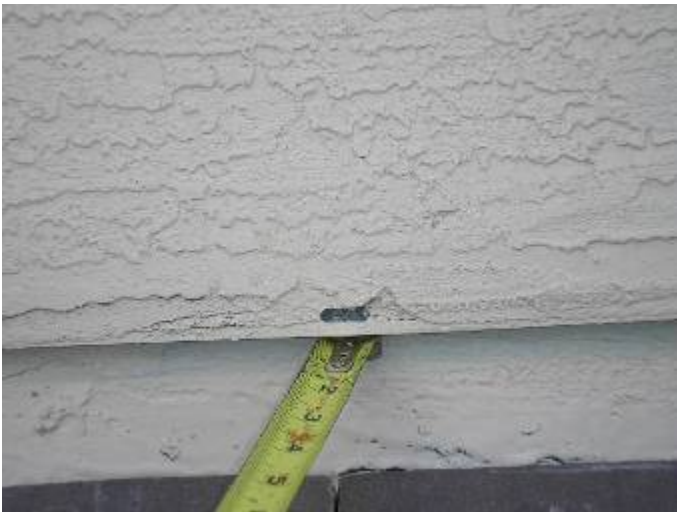
There is missing stucco outside the 2 nd floor north side exterior wall. §13-606.1.ABC.1.2, §1403.1.3.
