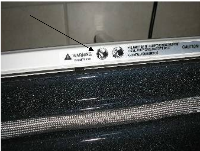
Note: the anti-tip device needs to be reinstalled when the range has been reinstalled after the mold repairs have been completed. §M304.1
