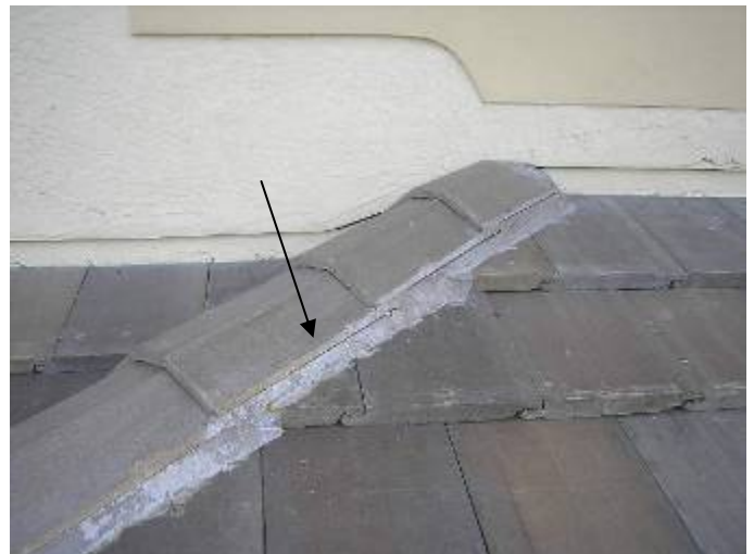
Some of the hip & ridge cap tiles do not appear to be correctly secured or bonded. §1518.8.5, §1518.8.11, 1507.4.5.2.1
