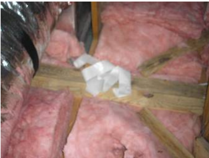
All scraps & construction debris should be removed from the attic.
