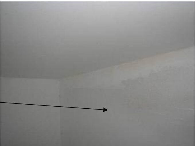
The drywall is not correctly finished or painted as required inside the master bathroom linen closet above the top of the door frame.
