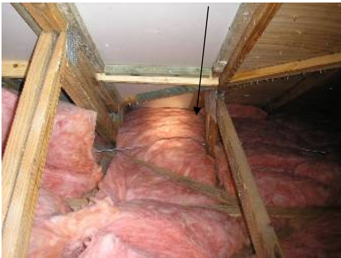
Some of the insulation is blocking the attic vent air circulation at the eaves. Baffle boards should be installed at all eave locations.
