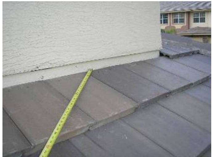
The roof wall abutments have not been correctly pointed up with mortar at the back patio. R118-3.13
