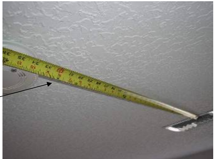
Some of the smoke detectors are located too close to the AC vents. A minimum of 3' clearance should be provided.
