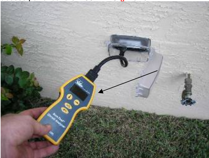
The rear GFCI protected receptacle outlets tested non-energized or no power.
