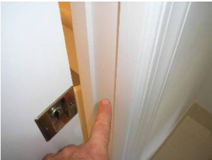
The latch did not engage correctly; the strike is not installed at the master bathroom pocket door. The door will not lock.
