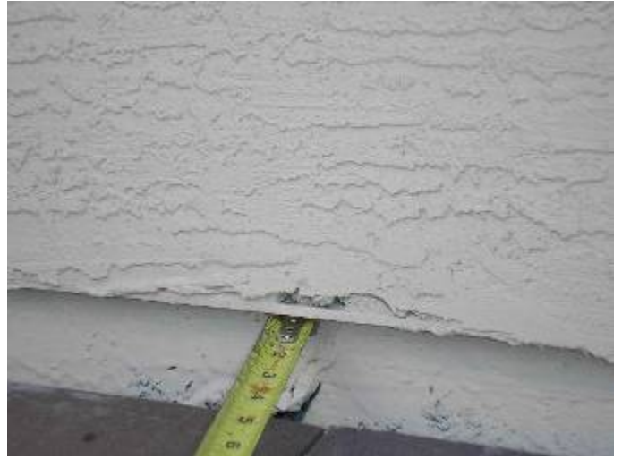
There is missing stucco outside the 2 nd floor north side exterior wall. §13-606.1.ABC.1.2, §1403.1.3.
