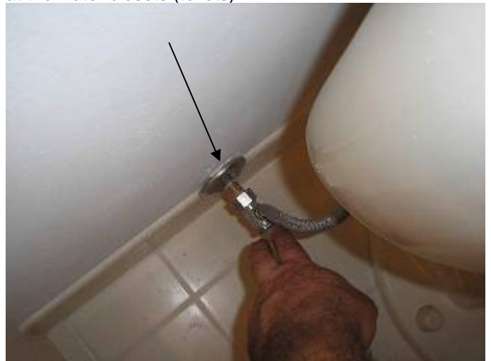
Some of the plumbing supply piping is loose & not correctly secured at the sink cabinets & behind the walls at the water closets (toilets).
