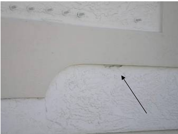
There is missing stucco above the garage roof tile at the 2 nd floor exterior wall. §13-606.1.ABC.1.2, §1403.1.3.
