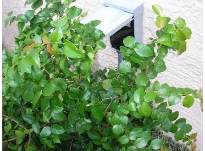
The landscape shrubbery is blocking access to the AC electrical disconnect box. 36" working space is required. 2002 NEC §110.26
