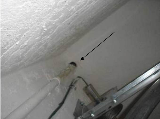
There are unsealed holes & openings in the drywall around the piping penetrations through the ceiling. The openings need to be sealed as required.
