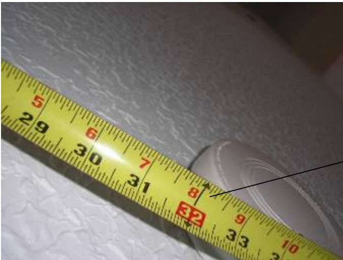
Some of the smoke detectors are located too close to the AC vents. A minimum of 3' clearance should be provided.
