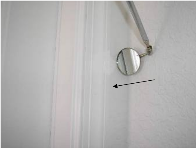
The side & tops of the garage/hall entry way door frame are not correctly sealed. §13-606.1.ABC.1.2
