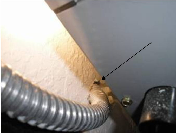
The AC mechanical closet is not completely sealed around penetrations through the walls & ceiling.
