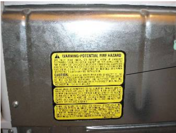
The thin aluminum foil dryer vent duct material is a fire hazard per CSPC & the manufacturer. See warning label on back of the dryer. §M304.1
