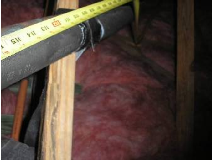
The AC refrigerant line is not correctly supported at 6ft intervals as required.
