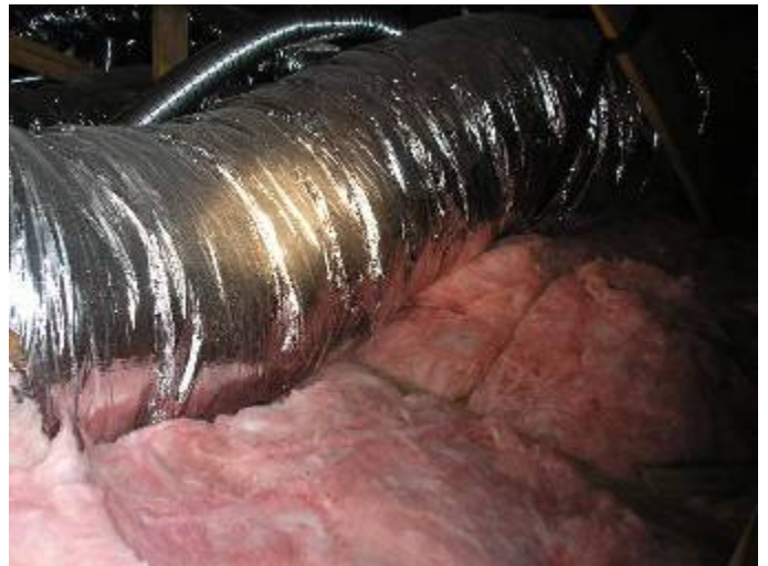
Some of the ductwork was not correctly supported off the attic insulation or other ductwork to prevent condensation & related problems. §M603.11, §M603.5.6.6
