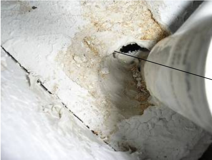
There are unsealed openings in the AC mechanical closet. §13-410.1.ABCD.3.7
