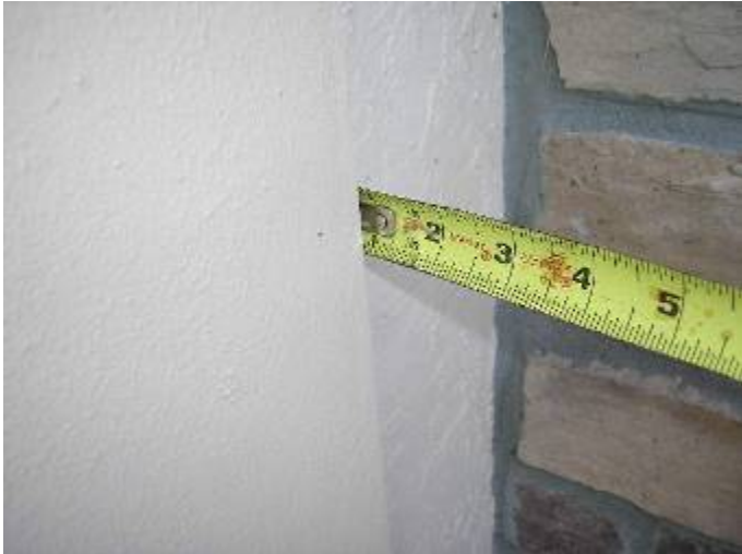
Some of the stucco work appears to be uneven & not the proper depth. ASTM C 926, §2504.2 §1403.1.3
