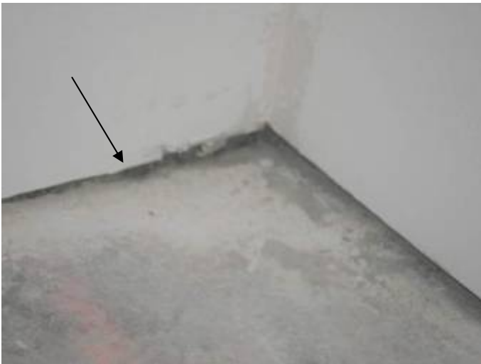
The walls are not sealed at the floor under the kitchen counters.
