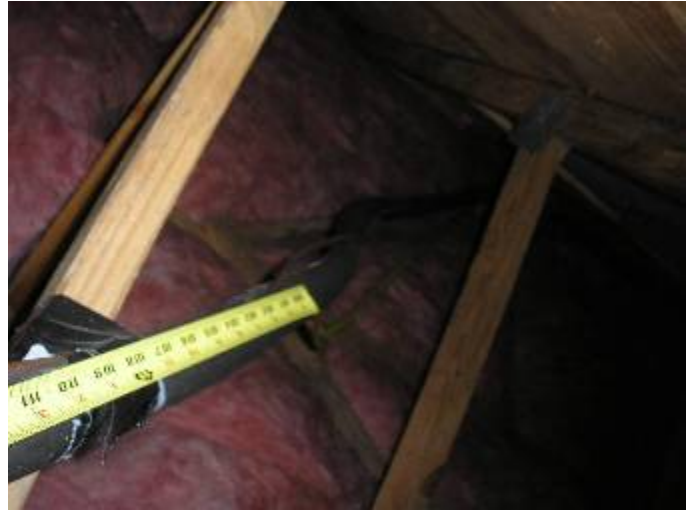
The AC refrigerant line is not correctly supported at 6ft intervals as required. §M305.4
