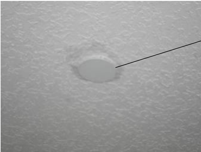
The fire sprinkler cap appears to be sealed in place & would not work in the event of an emergency.
