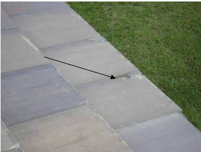
There should not be any broken tiles on the new roof. The tiles need to be removed & replaced; not "glued" back together.
