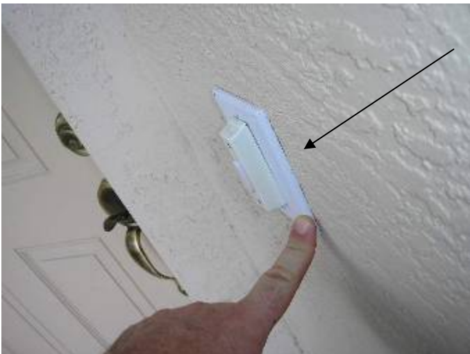
The door bell cover is not sealed as required. §13-606.1.ABC.1.2
