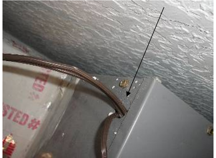
The grommet is not installed around the thermostat low voltage line at the top of the AC air handler. §M304.1 See the manufacturer's installation instructions.
