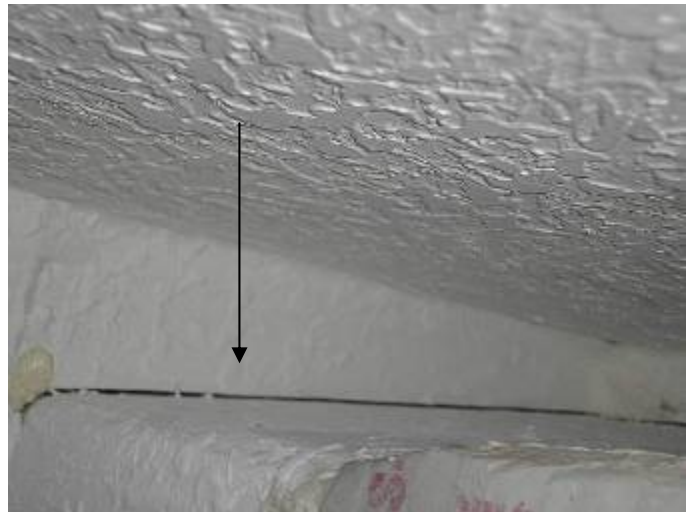
The drywall is not correctly sealed around the ductwork in the AC mechanical closet. §13-410.1.ABCD.3.7
