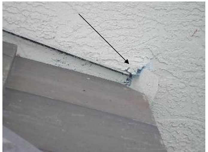
There is not enough stucco to seal the wall around the roof abutment "kick out" flashing at the back of the house. §13-606.1.ABC.1.2, §1403.1.3.
